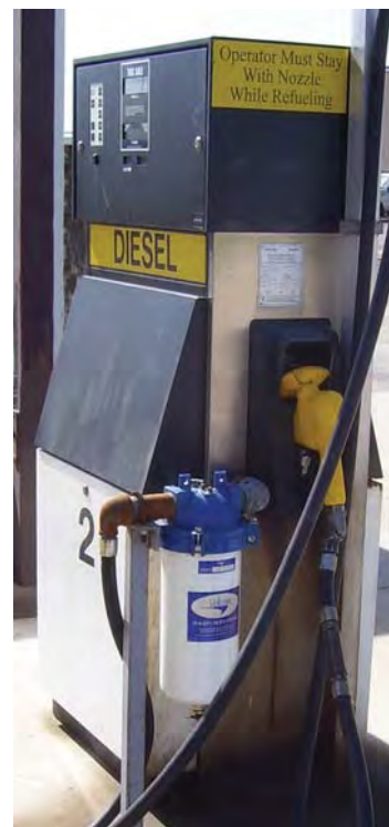
VF-61 connected to a diesel fuel dispenser
