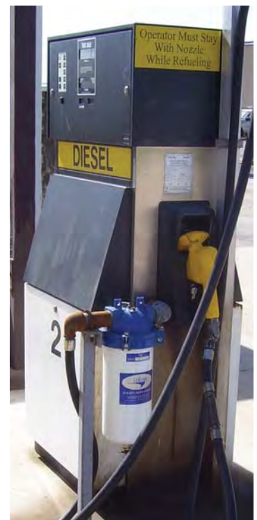
VF-61 connected to a diesel fuel dispenser
