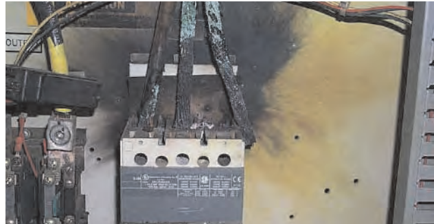
Photo 3, Arcing Caused by Loose Input Contacts
