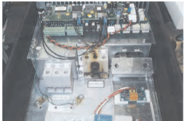
Photo 4, Arcing Caused by Loose Output Contacts
