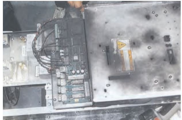
Photo 1, Fan Injecting Dust into Drive Enclosure
